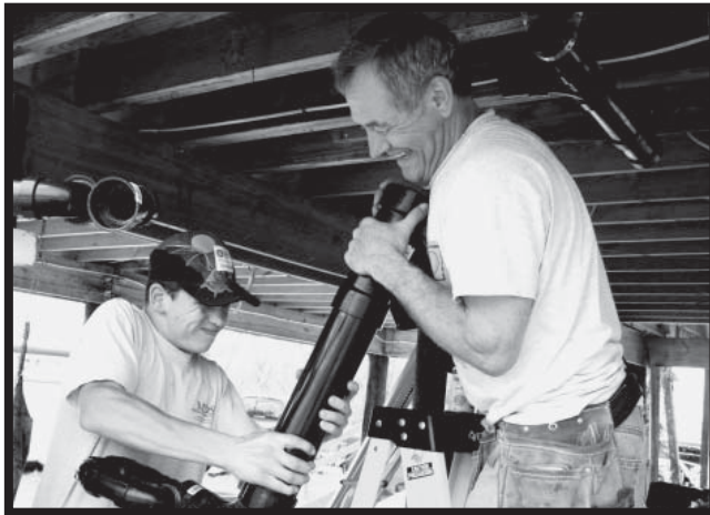
VOLUNTEERS IN LOWER PLAQUEMINES PARISH, DIAMOND, LOUISIANA INSTALLING NEW PIPES IN A HOME DAMAGED BY HURRICANE KATRINA
