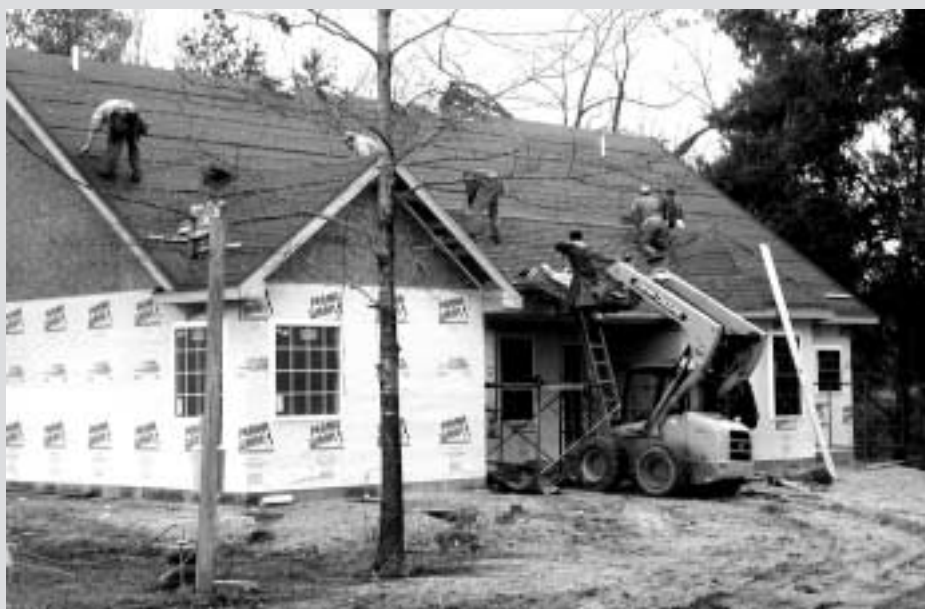
Volunteers work on the MDS “Hands On House” in Columbus, Mississippi. The completed home will be landscaped and sold by a realtor. Proceeds from the sale will benefit MDS binational, Region II and the Mississippi Unit.
