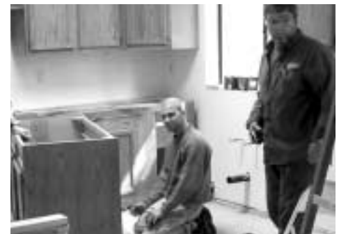
Mark Hochstetler and Freeman Hershberger install kitchen cabinets in the Pinedale home.
