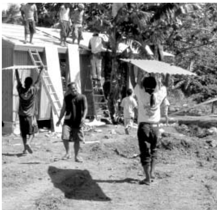
Under the direction of MDS volunteers from North America, Chuukese laborers rebuild a storm-damaged home in Micronesia.
