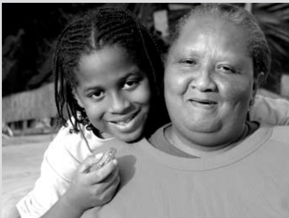
Cora Henning and her grandson sit on the foundation of an addition that Mennonite Disaster Service is building to replace a room that was blown away from her home during the Jackson tornado.
